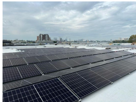
Shurgard Stadionweg store in Rotterdam. a new building (certified with BREEAM "Very Good") of a total of c. 13,000 sqm, has been equipped with 420 sqm of PV panels placed on the roof.
